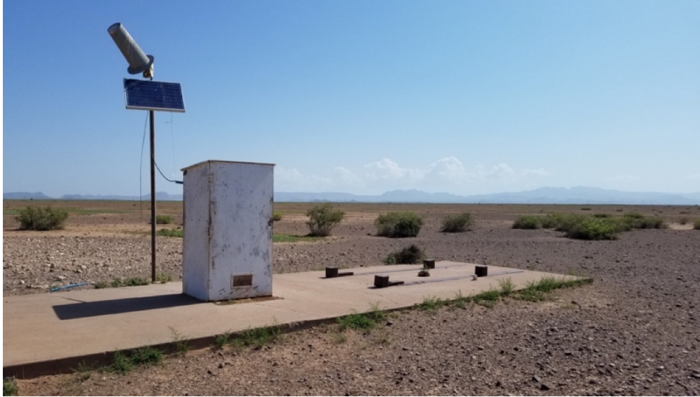
Figure 22. Presidio recorder well location.
