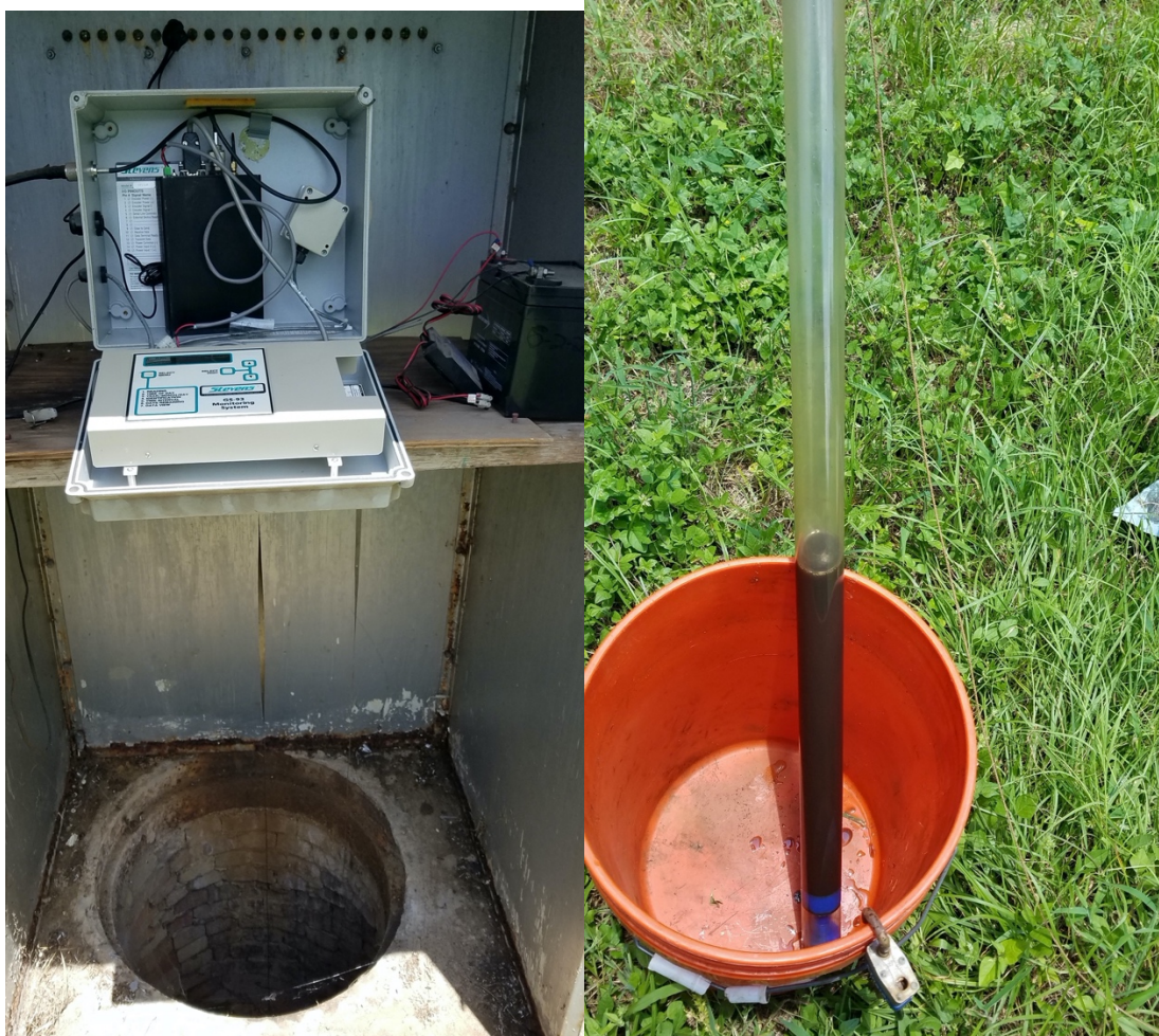
Figure 12 (left). Dallas recorder well, showing uncovered well opening Figure 13 (right). Oil sample collected from Dallas recorder.
