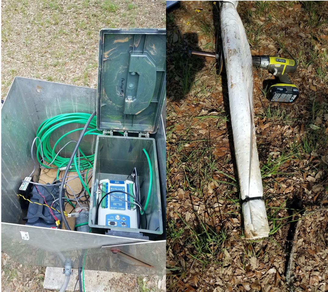
Figure 9. Comal recorder well head, showing excess cable coiled in shelter.
