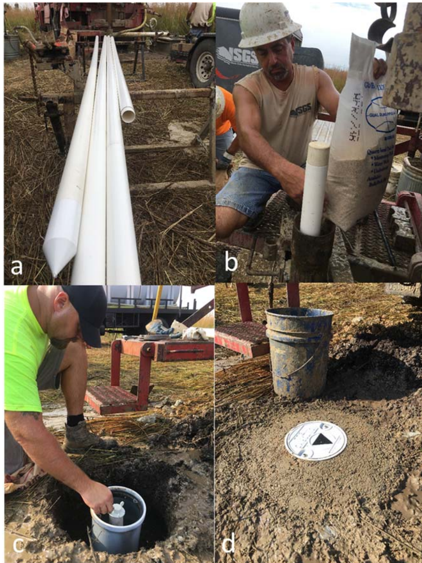
Figure 8. (a) 2-inch PVC casing and screen ready for installation, (b) installing sandpack material, (c) well casing with lockable cap and (d) completed wellhead protector.
