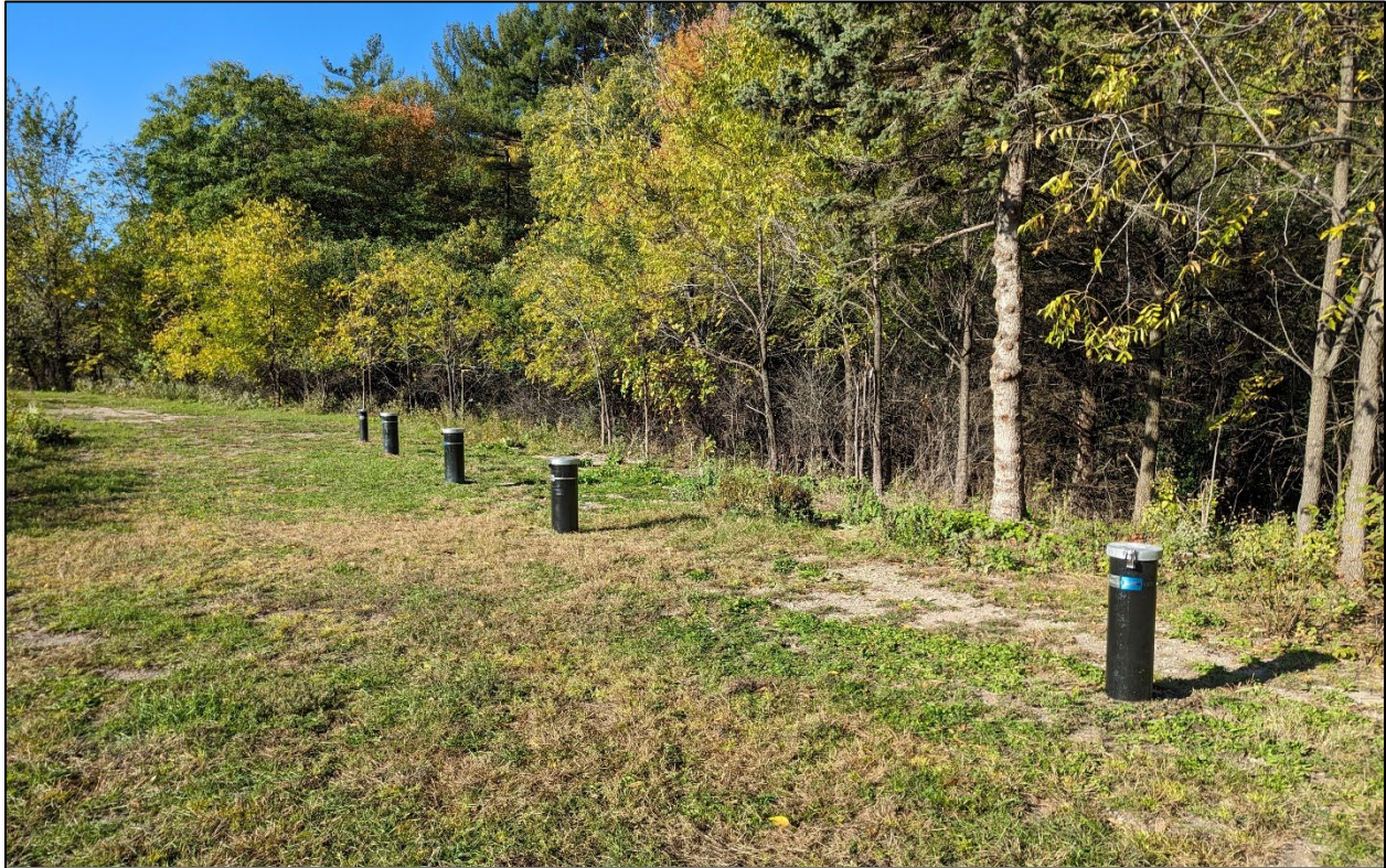
Figure 1: A site photograph showing the five new groundwater observation wells that were installed as part of this project.
