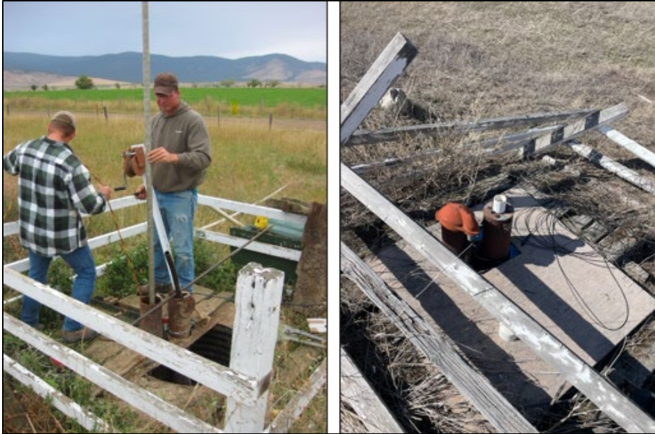
Figure 3. MBMG-6283. The drop pipe could not be completely removed, preventing a downhole camera survey and sounding; the well was surveyed.
