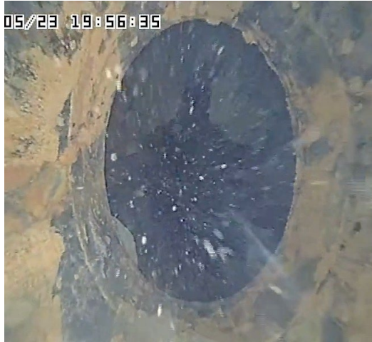
Figure 14. Downhole image of the bottom of the casing at 147 ft.
