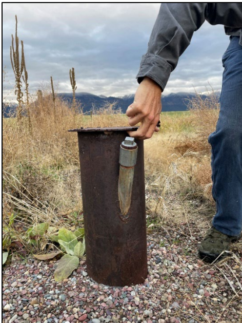
Figure 4. MBMG-76048. The well cap is welded on, preventing a downhole camera survey and sounding; the well was surveyed.
