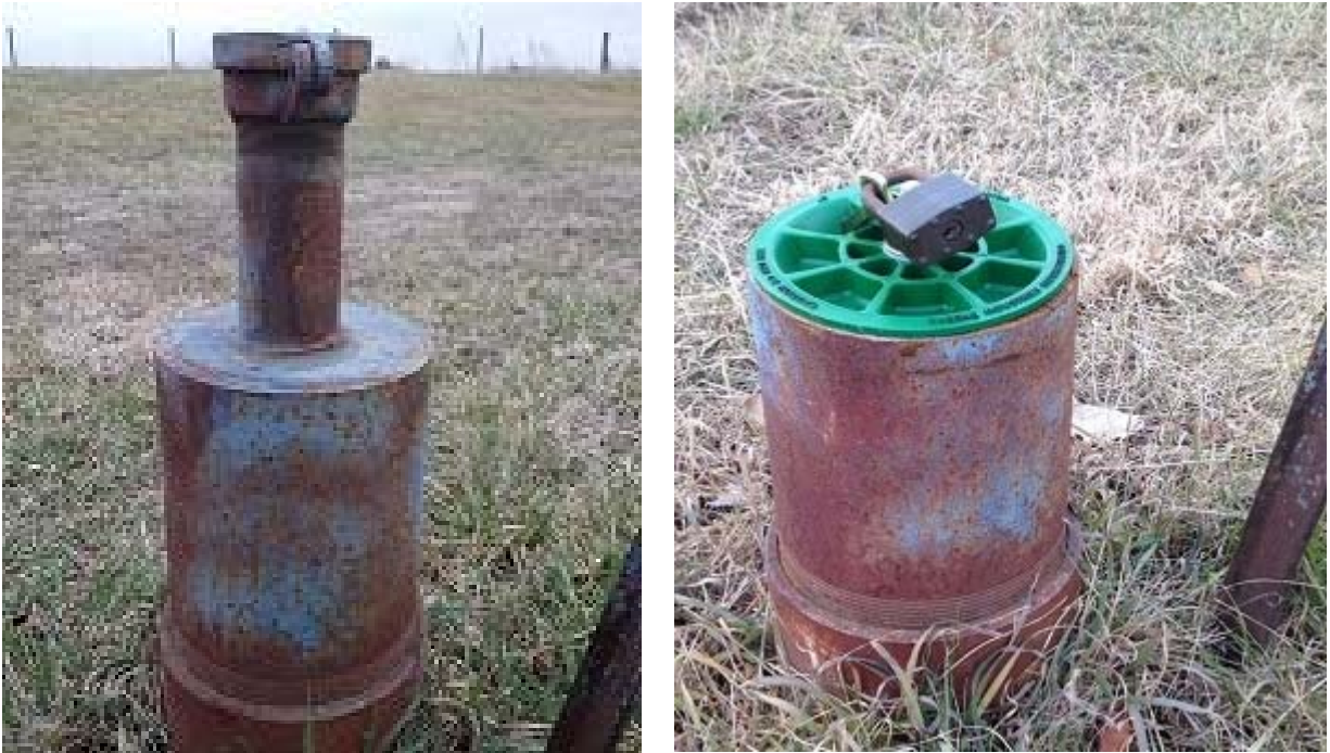
Figure 2. A well cap on an IGS network well before (left) and after (right) modification.
