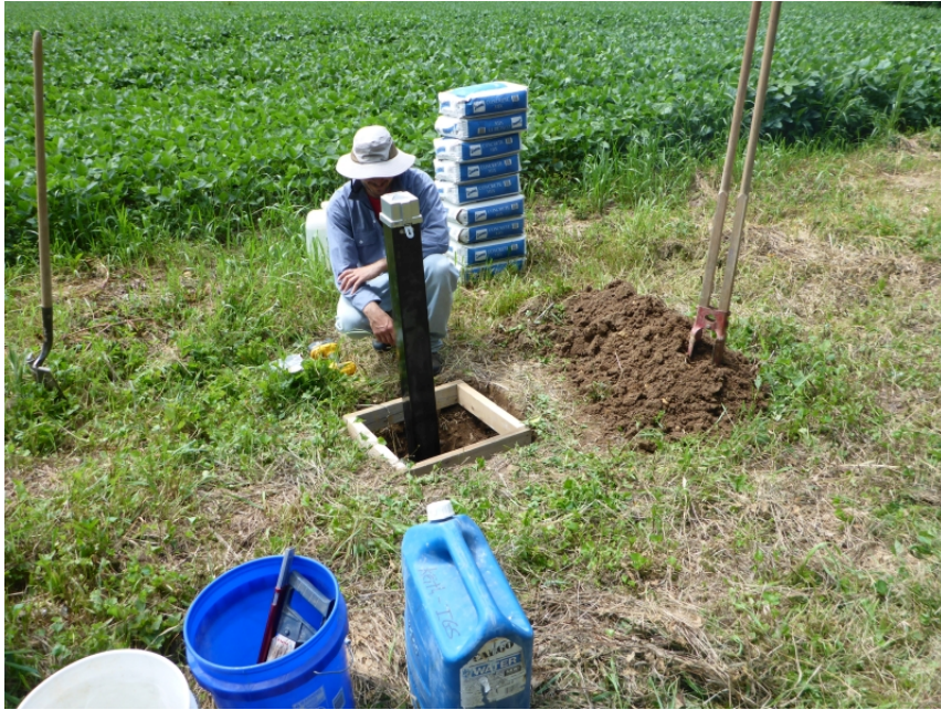
Figure 4. Image showing IGWS personnel installing a protective well cover at the Rushville_S monitoring site.
