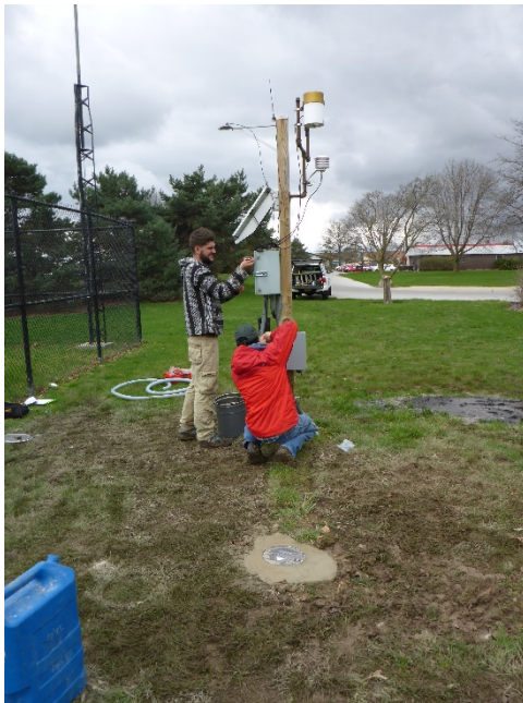
Figure 5. Image showing IGWS personnel installing a flush-mount protective well cover at the Muncie_N monitoring site.
