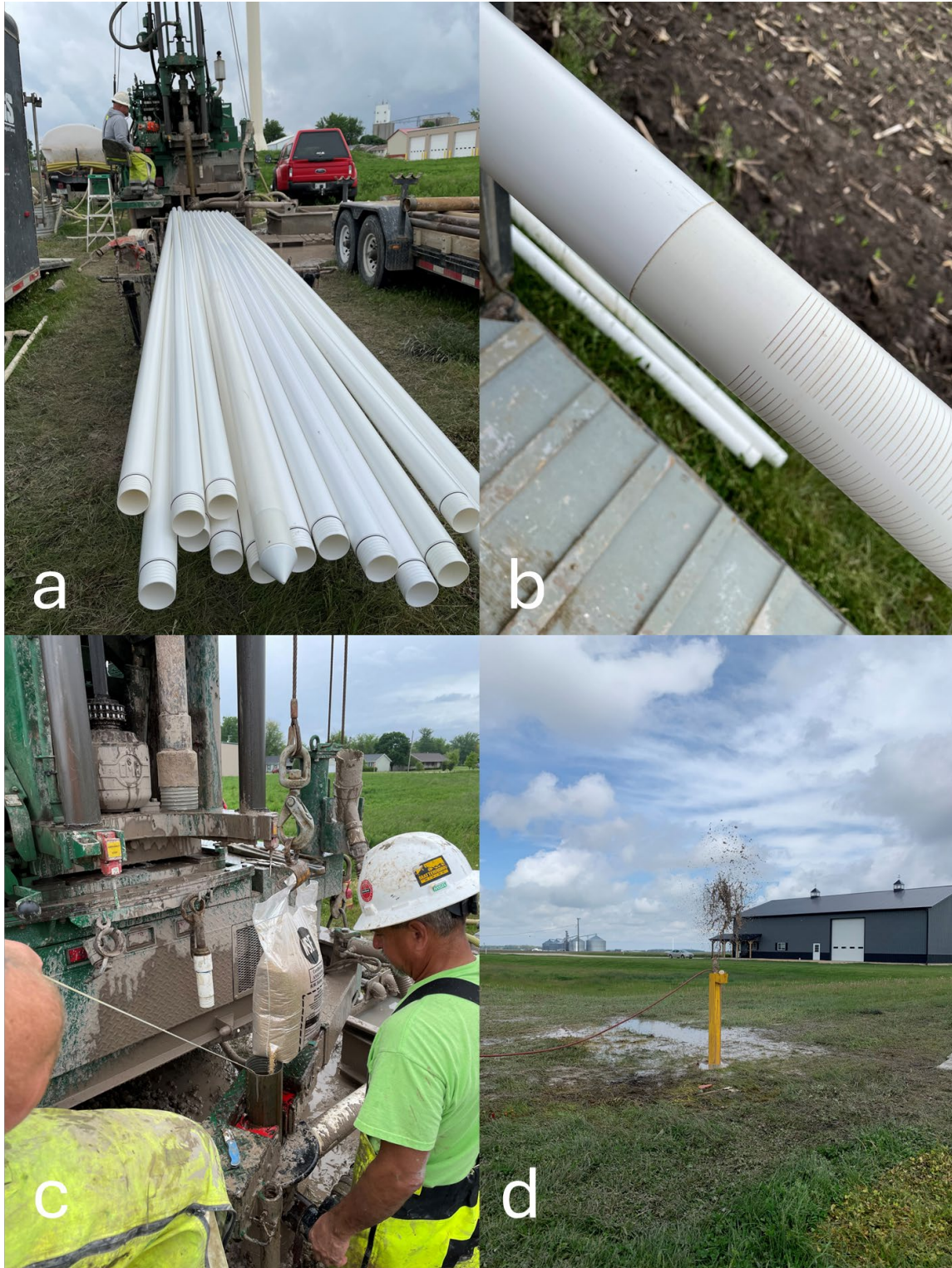
Figure 7. (a) 2-inch PVC casing and screen ready for installation, (b) well screen, (c) installing sand pack (d) completed wellhead protector during air-spurge well-development. All photos are from the SUBL-21-01 site at Sublette, Illinois.
