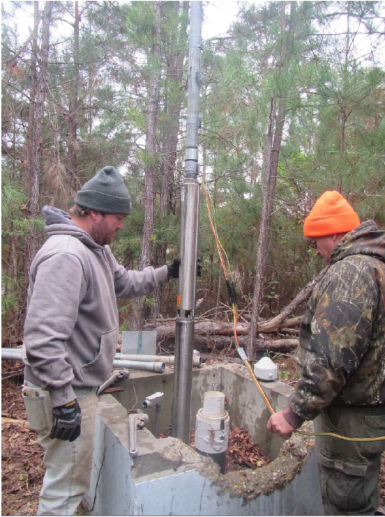
Figure 7.—Submersible pump installation in well MTG-6, GSAL111889, Montgomery County, Alabama, prior to aquifer test conducted on November 12, 2023.
