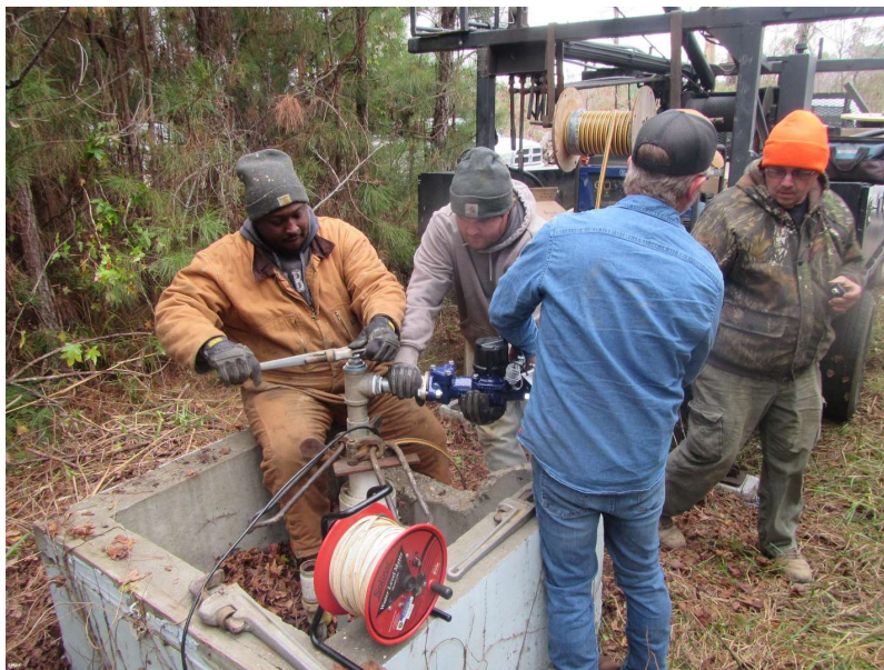
Figure 8.—Orifice installation at well MTG-6, GSAL111889, Montgomery County, Alabama, prior to aquifer test conducted on November 12, 2023.
