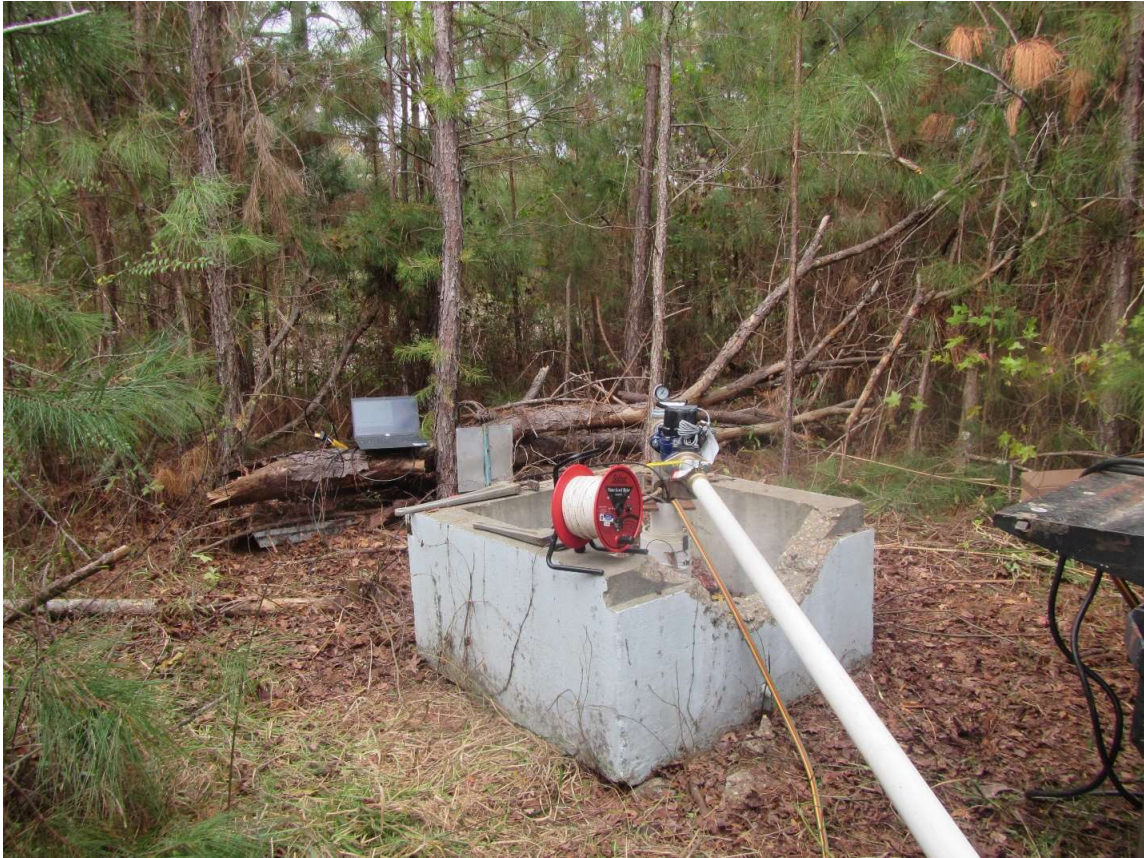
Figure 9.—Final orifice assembly and discharge pipe at well MTG-6, GSAL111889, Montgomery County, Alabama, prior to aquifer test conducted on November 12, 2023.
