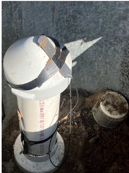
Figure 11. Trend well GSAL 125719 (MAG-1) after repairs. Photo illustrates 4-inch PVC casing and mounting collar installed during repairs.
