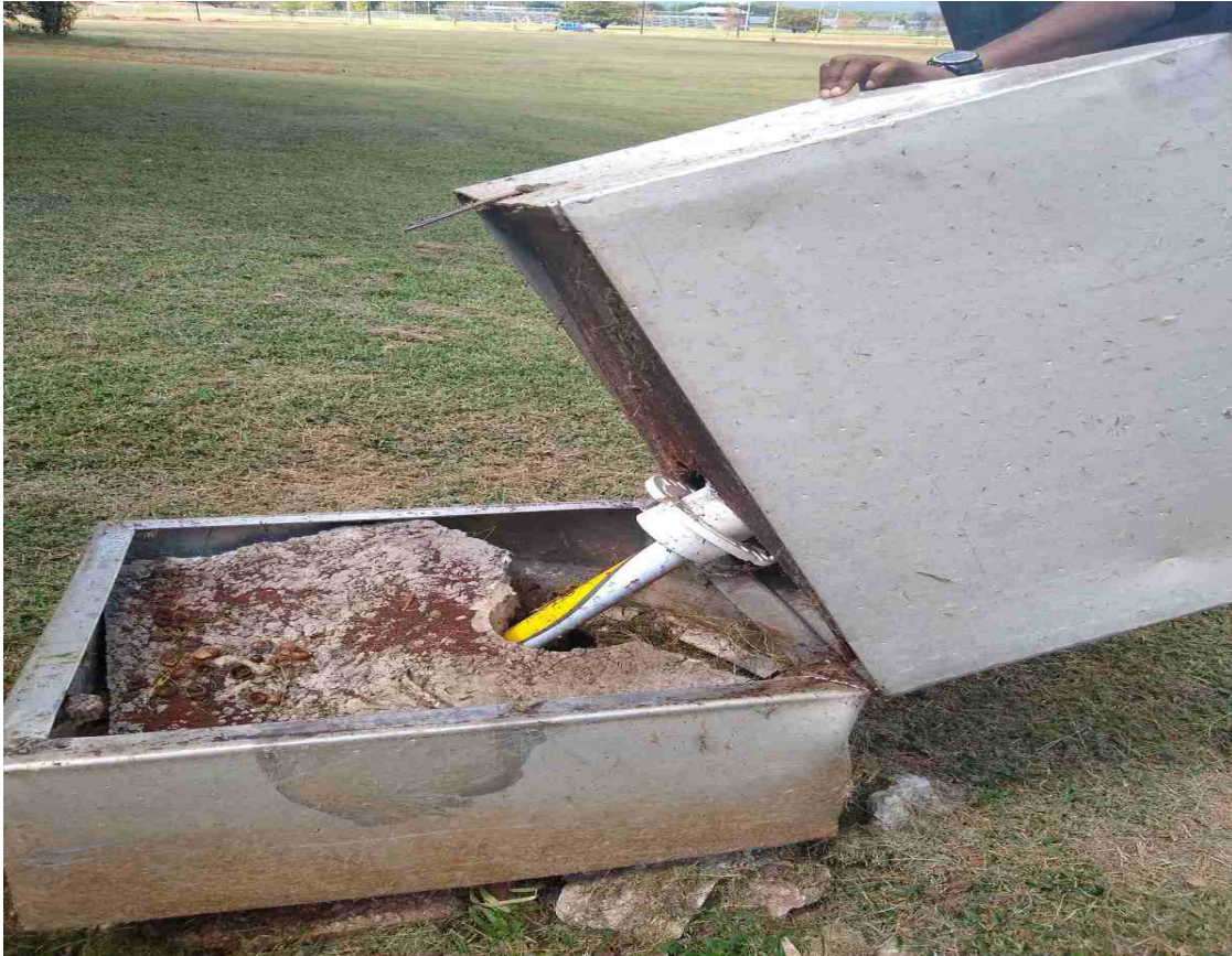
Figure 8. Trend well GSAL 125687 (MAD-2) prior to repairs.
