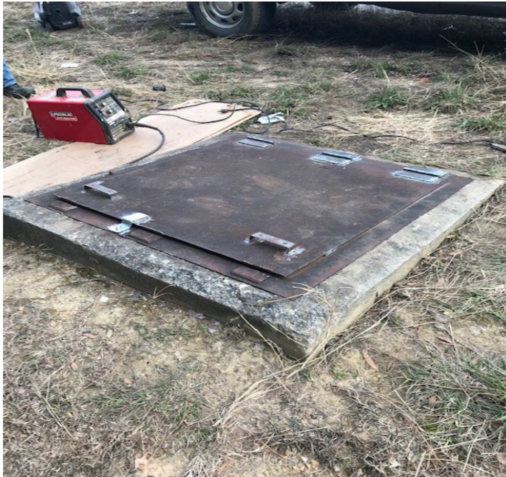
Figure 6. Trend well GSAL 125344 (JEF-1) after repairs. Photo illustrates three new hinges, lock hasp, and handles installed during repairs.
