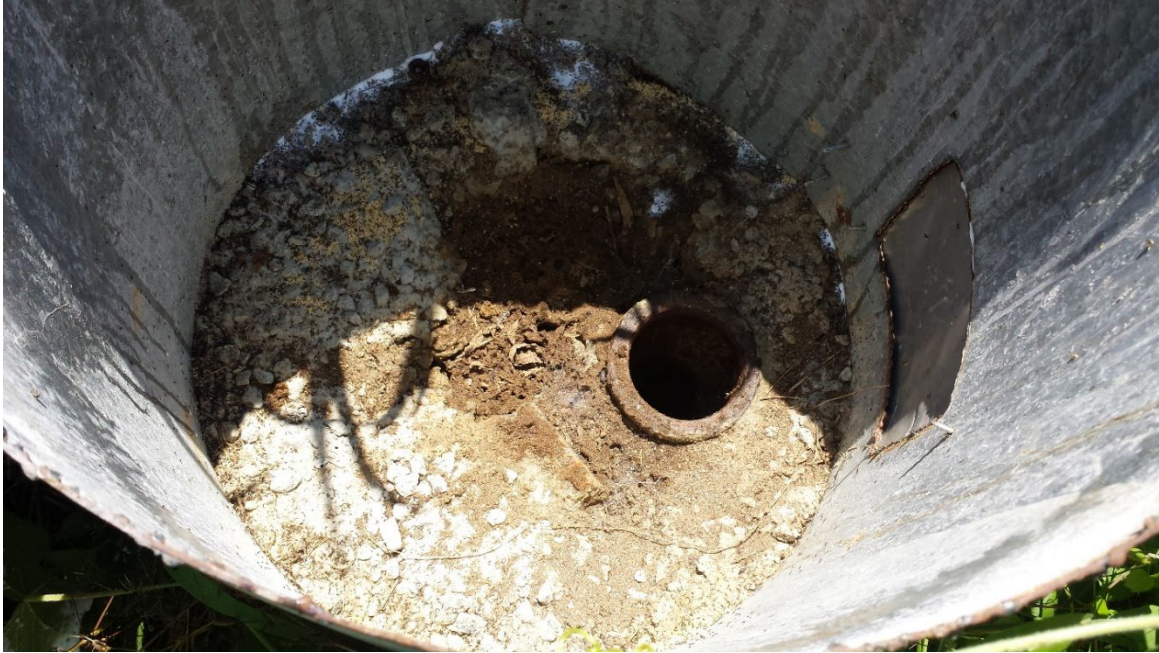
Figure 10. Trend well GSAL 125719 (MAG-1) prior to repairs.
