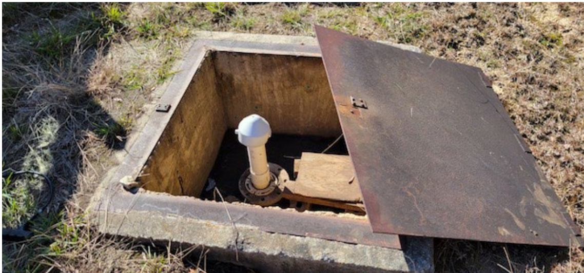
Figure 5. Trend well GSAL 125344 (JEF-1) prior to repairs. Photo illustrates broken hinges and lock hasp.
