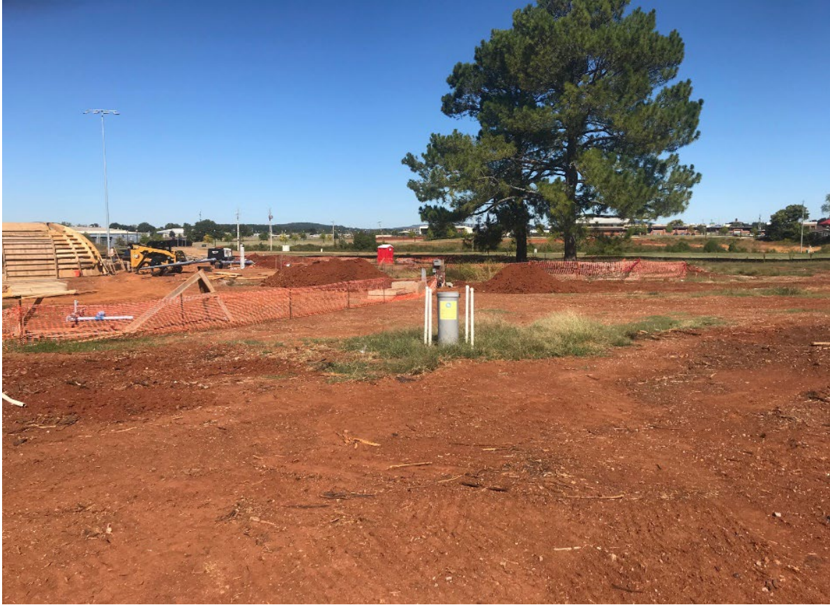
Figure 9. Trend well GSAL 125687 (MAD-2) after repairs. Photo illustrates PVC surface casing, locking cap, and guard posts installed during repairs.
